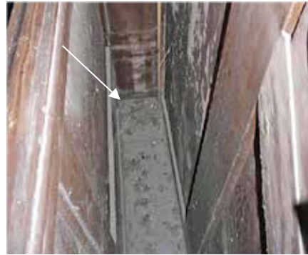
Accumulated debris between stair and pew. Note ghost of earlier partition on the wainscot. This represents an earlier pew that pre-dates the stair.
