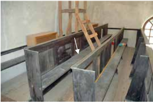
Gallery pews missing caps and back panels
